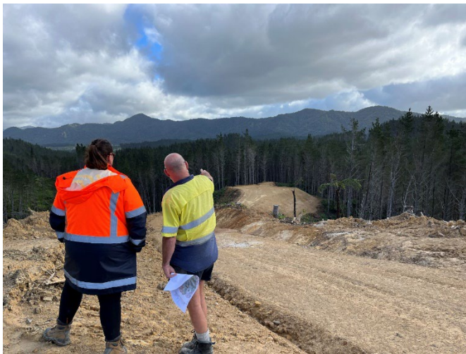
Figure 1: SFNZ describes the earthworks process to new Northland Regional Council compliance staff at a non-operational site.
